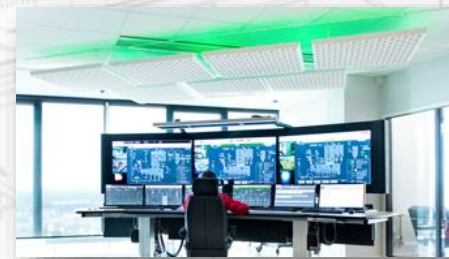
Distributed control systems
